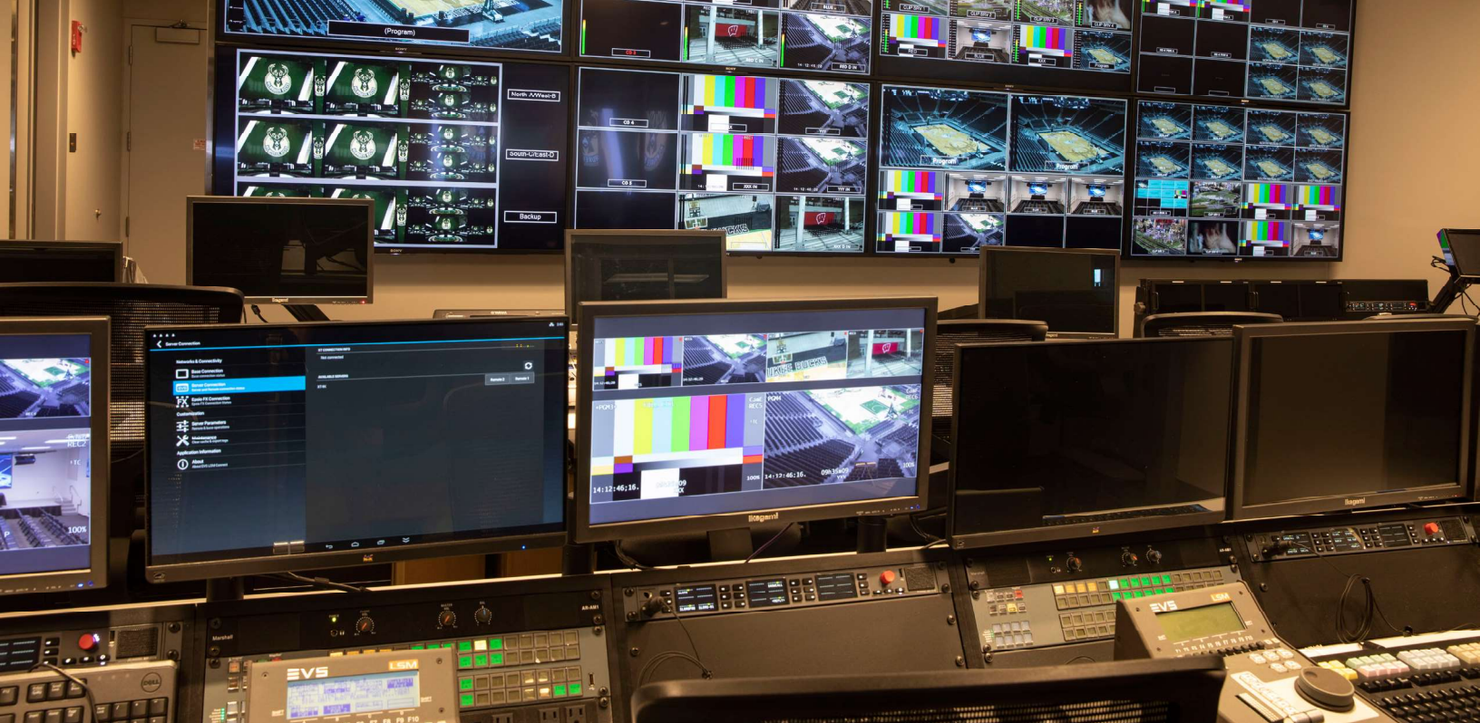
Video Control Room
